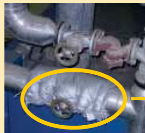
Non-isolated valve above Isolated valve in circle
